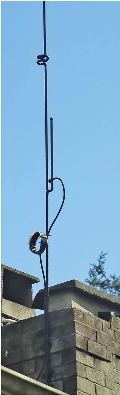
Figure 4 — The roof-mounted saxophone antenna. The coiled choke balun shown is a poor choice. A much better solution would be two to three turns of the coax through a mix-31 toroid.
